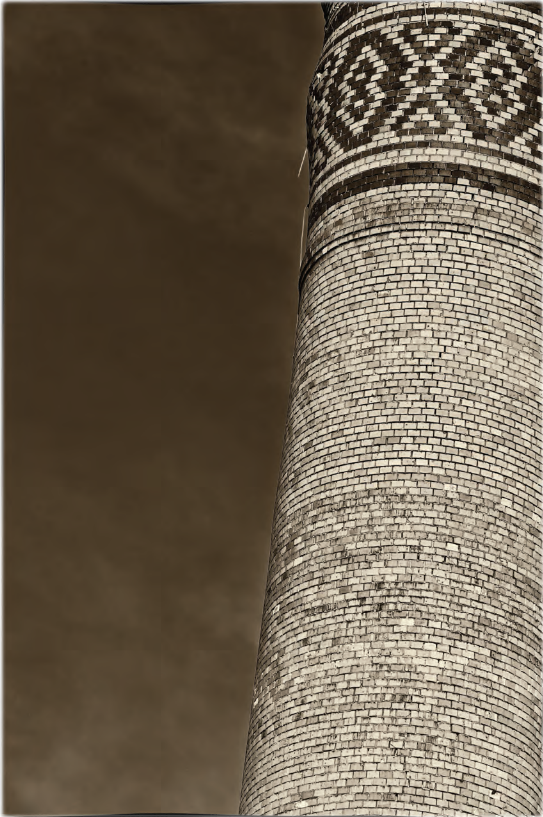
Detail, top portion, showing brick patterning and bulge from winter damage, American Thread Mills Bldg No. 2 smokestack, Willimantic, Conn.
