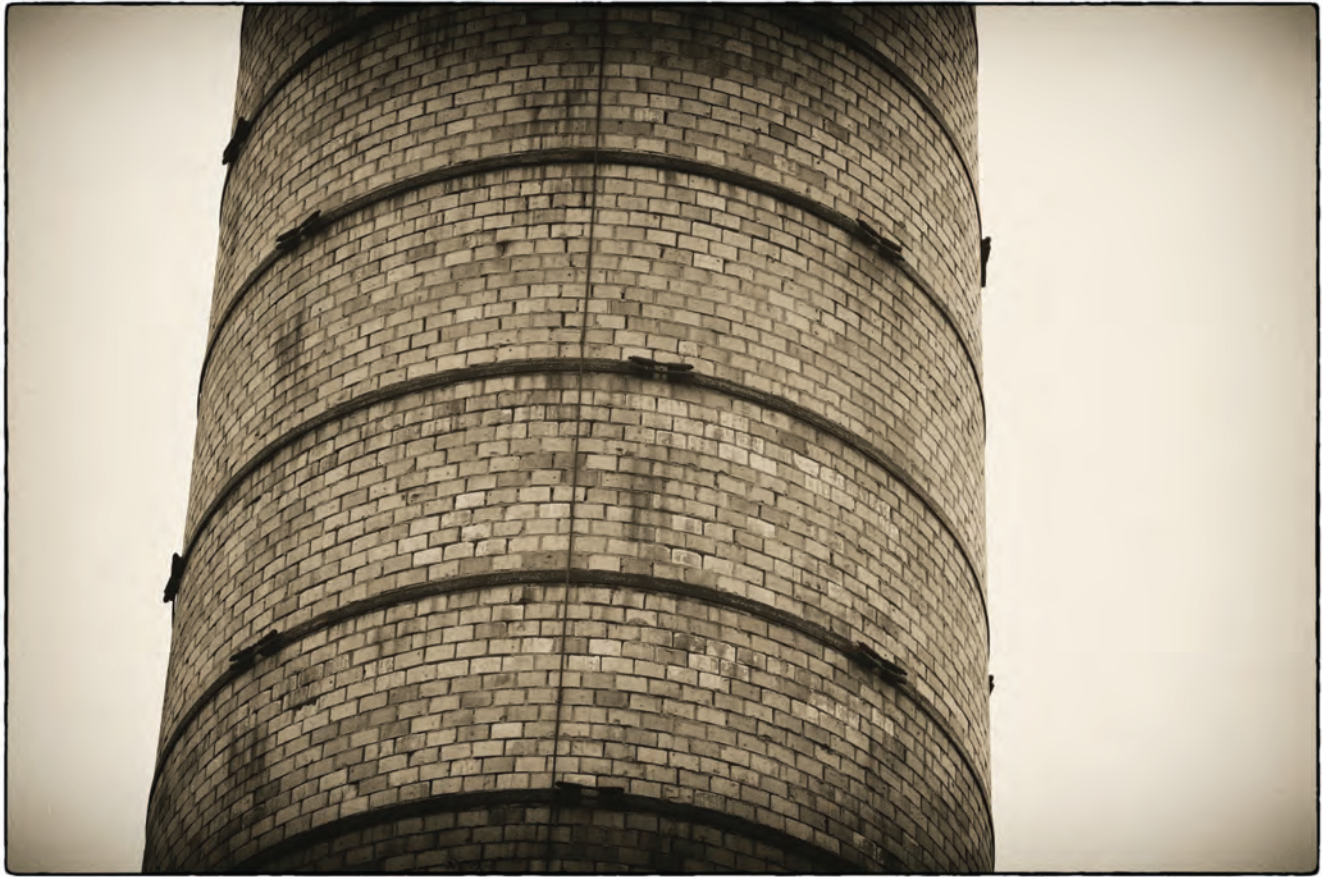
Detail, central portion, showing steel retaining bands, American Thread Mills Bldg. No. 2 smokestack, Willimantic, Conn.
